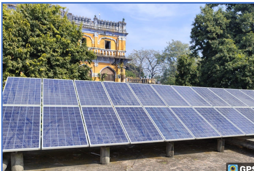
Figure 2: Solar power plant in campus
